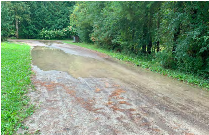
Figure 3: Poorly drained segment of Udora gravel road
